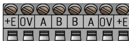
Picture 6 Terminal connection of bus line cables
