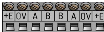
Picture 4 Terminal connections of power supply cables
