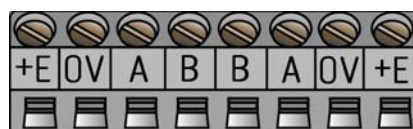
Picture 6 Terminal connection of bus line cables
